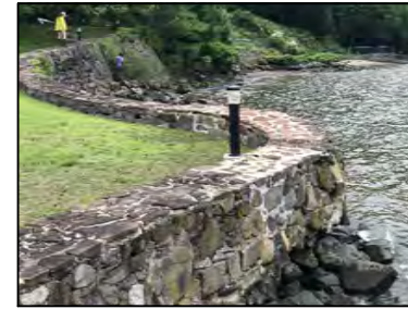
SEAWALL CONDITIONS AT LOW TIDE
