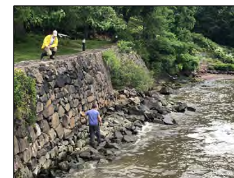
SEAWALL CONDITIONS AT LOW TIDE
