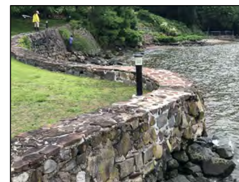
SEAWALL WASHOUT AND RIP-RAP
