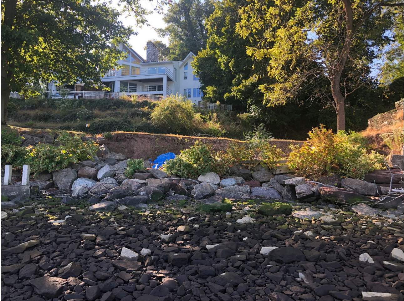
Photograph 1: Eroded seawall to be reconstructed – facing north.
