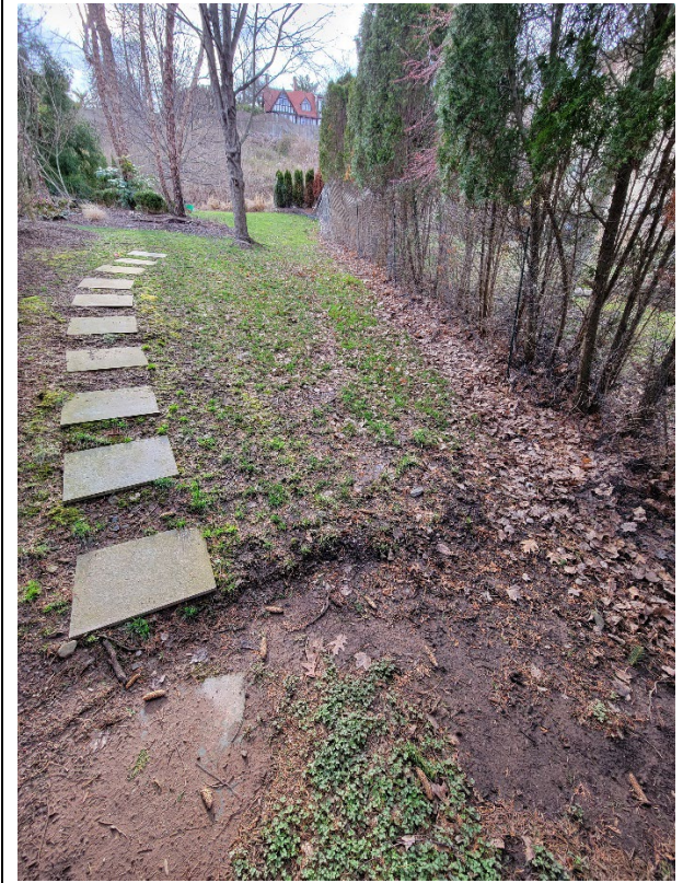
Drainage issue, northern side
