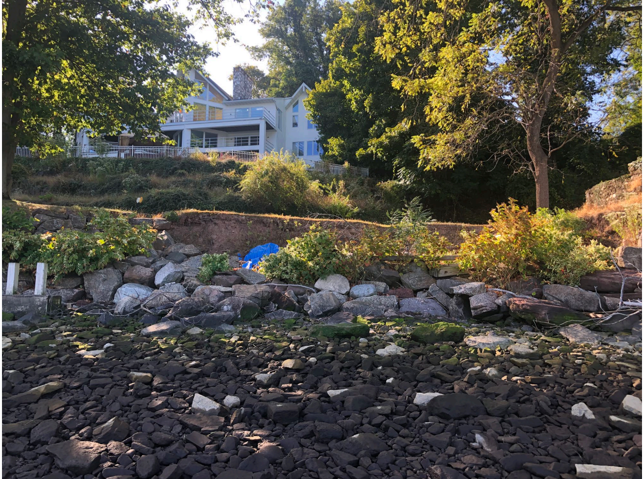
Photograph 1: Eroded seawall to be reconstructed – facing north.
